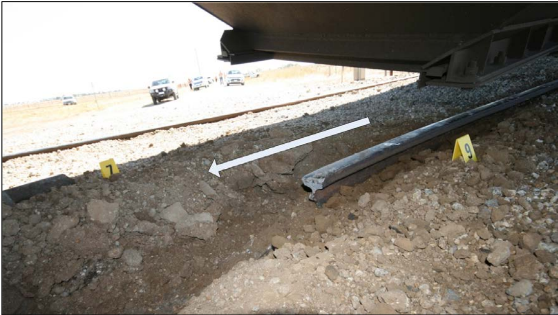
Figure 2: The broken rail within the level crossing
