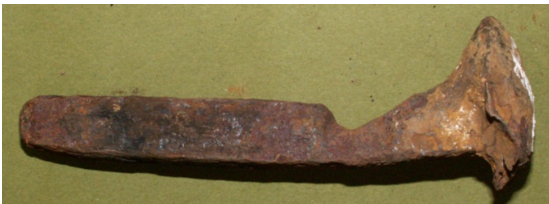
Figure 12: Typical corroded and worn dog spike
