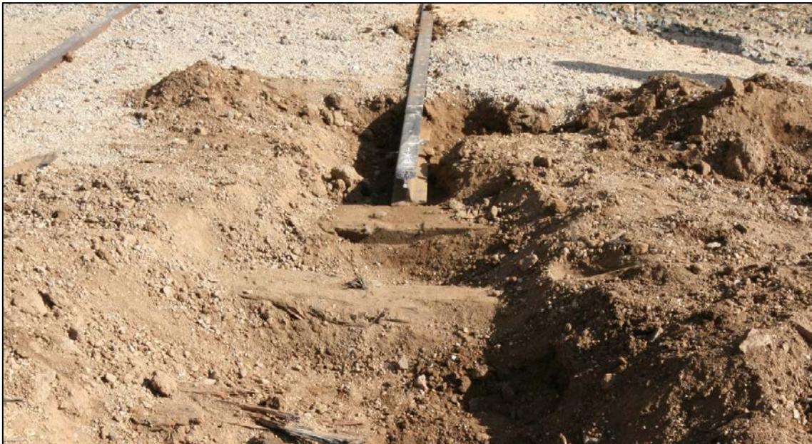
Figure 7: Point of derailment following excavation
